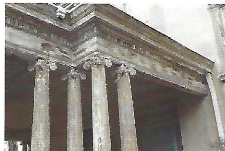
▲ Careful prep work was key to restoring this beautiful early-twentieth century home.
